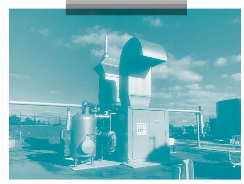
The new cogeneration unit powered by biogas at Colac Water Reclamation Plant.
