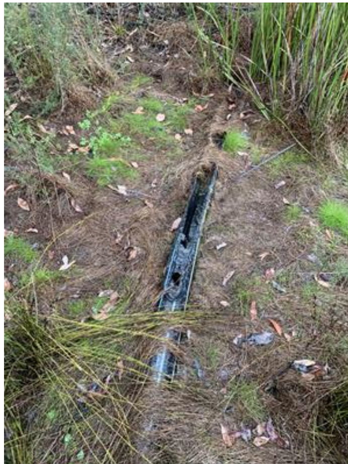
Image 25. Burnt plastic pipe located in the Sedge Wetland in the offset site (Figure 2, HHa assessment point 2d) (May 2023).
