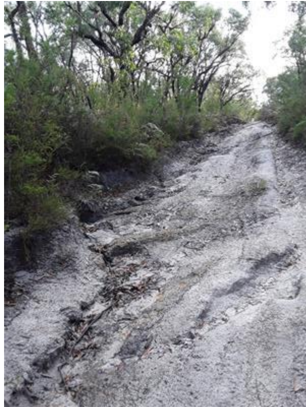
Image 8. An example of one of multiple areas of erosion and sandy soils on internal tracks in the offset site (May 2023).
